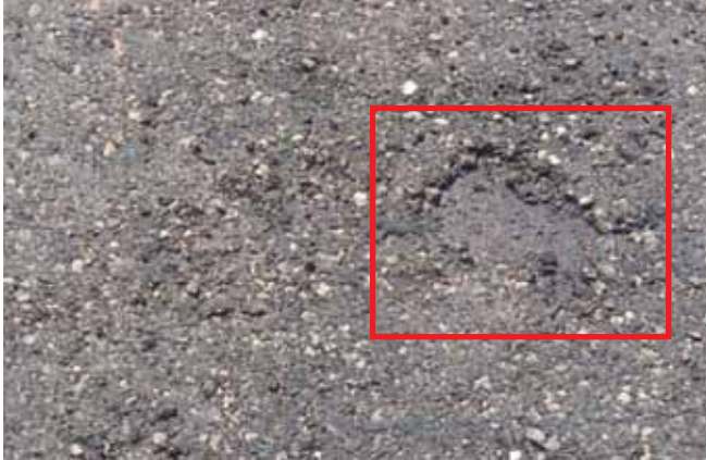
Mark the area of the pothole
