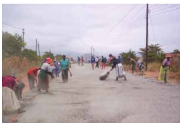
Un-even spreading of aggregate
