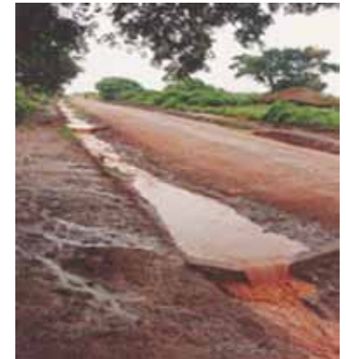
A functioning scour check
